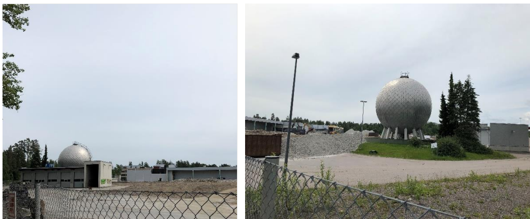
Figure 3. Demolition works in Kera started in the beginning of 2022. Source: City of Espoo
