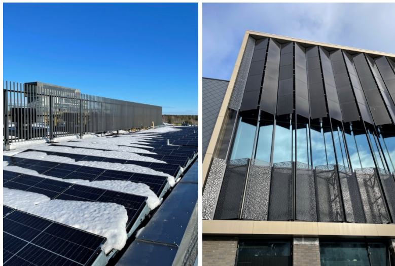
Figure 4. PV panels embedded in the facade and on the roof in Lippulaiva shopping center. (Source: Citycon).
