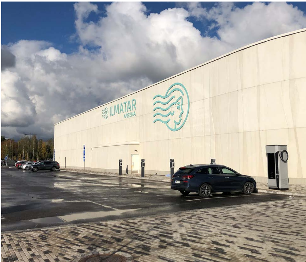
Figure 49. Installed EV chargers in Ilmatar arena, 8x22kW AC chargers and 1x160 kW DC charger. (Source: Siemens)
