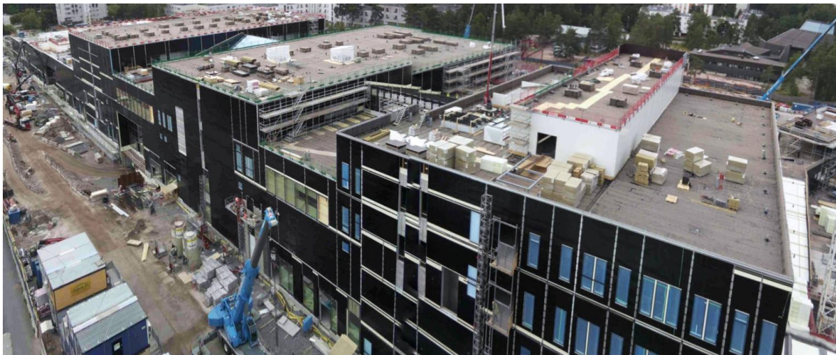
Figure 2. Lippulaiva architecture picture as it will be when ready (above) and picture of construction site from 12 th of August 2020 (below).
